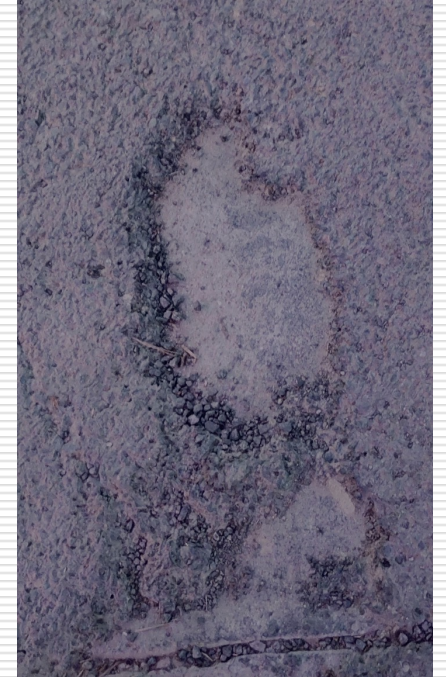
Pothole in front of Hall-1
