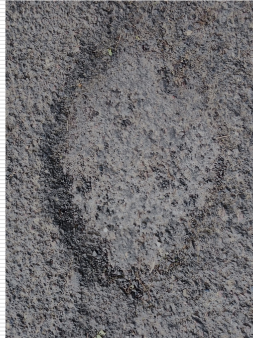
Pothole in front of Hall-2
