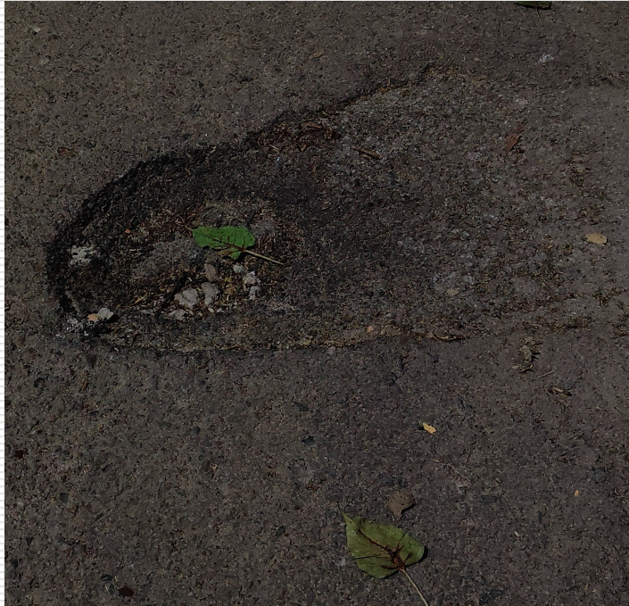
Pothole on road in front of campus e-shop
