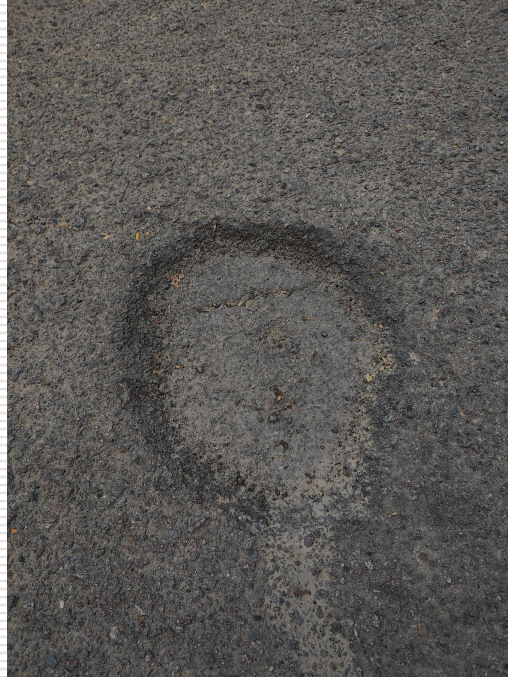
Pothole near the BSBE building, close to academic gate 3
