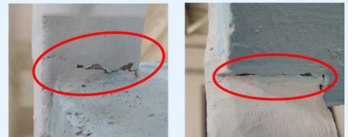
Observed damages at joints
